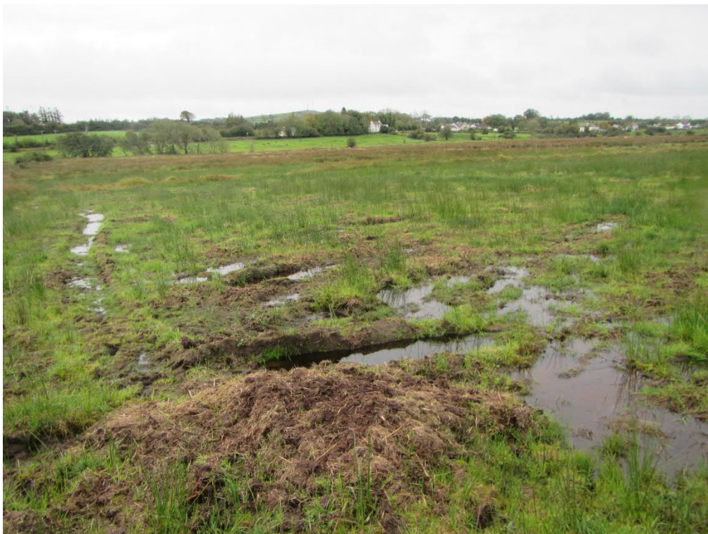
Photograph 14.8 Extremely wet ground within the Proposed Road Development to the north of the Abbart River.
