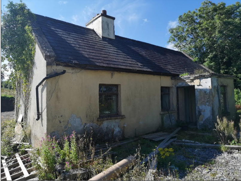
Plate 1. Building BLD01. Renovation works are planned. Classified as having 'Moderate' bat roost potential
