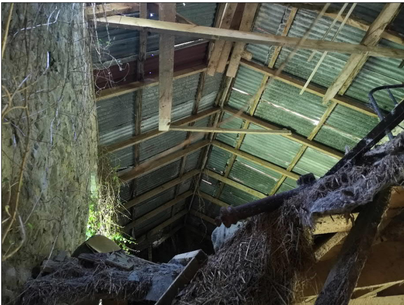
Plate 8. Interior of Building BLD04 showing. Access to the loft was not possible due to collapsed floor
