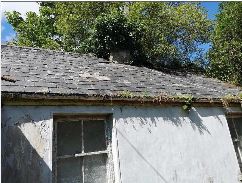
Plate 6. Intact roof on Building BLD03 increasing the possibility of this building being used by bats
