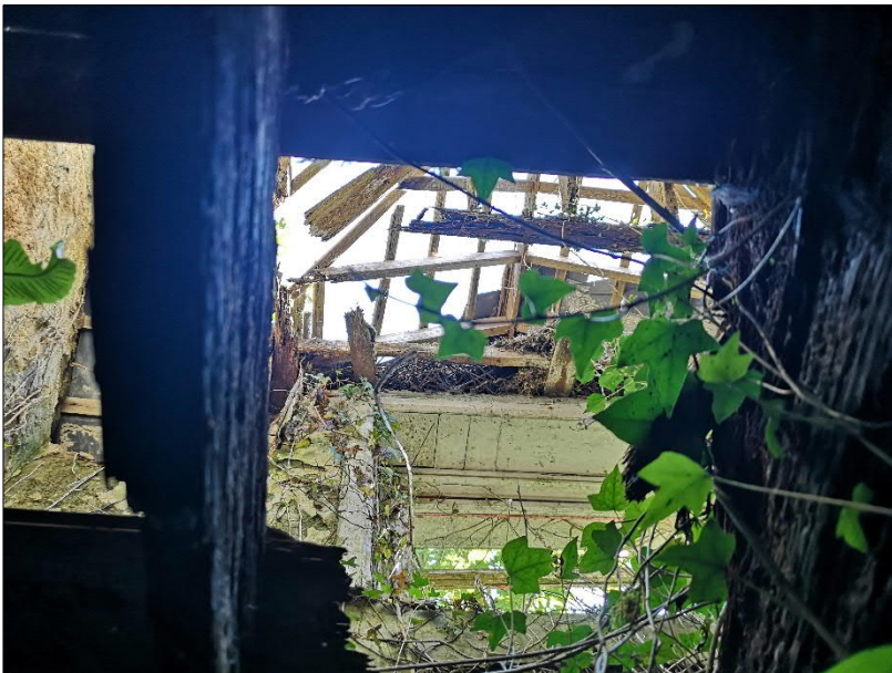
Plate 10. Much of the roof of Building BLD05 is missing, reducing bat roosting opportunities.
